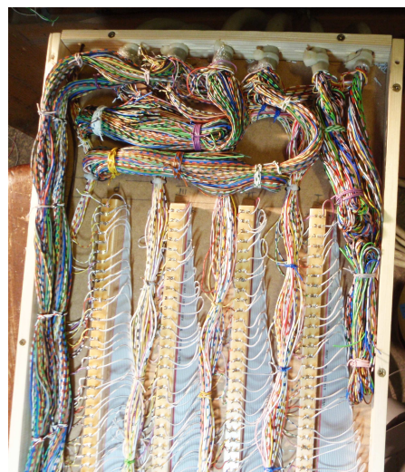
Figure 7: Finished distribution. The ribbon cable is facing towards the bottom.
