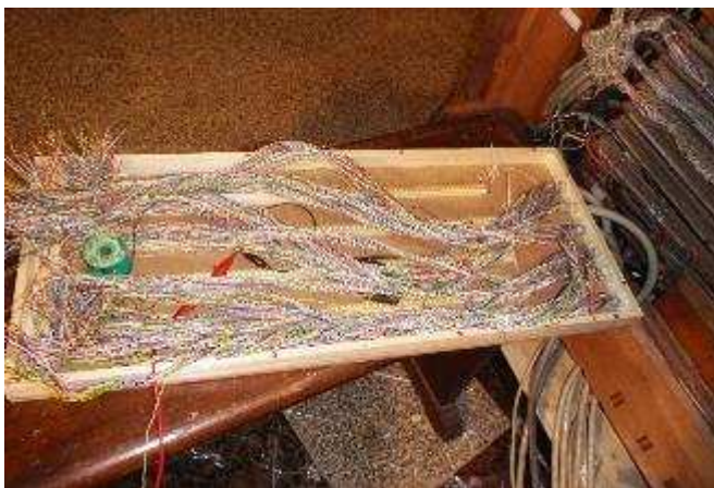
Figure 8: One of the 3 electrical distribution boards with the cables from the console
